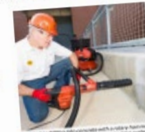
Worker using handheld drill with a HEPA-filtered vacuum system equipped with a shroud and dust collection system.
