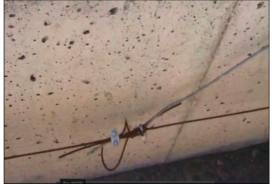
Rusted cable repaired by attaching new cable to old rusted piece
